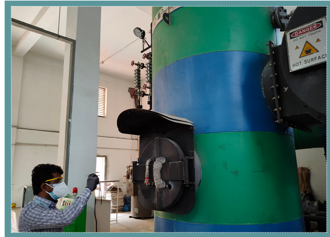
An RSC engineer conducting a visual inspection of a solid fuel boiler combustion chamber. Photo credit: RMG Sustainability Council (RSC)
